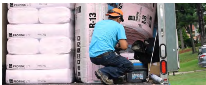
Workers prepare for a home insulation retrofit in Baltimore, Maryland. Adding insulation to a home can help maintain consistent temperatures and a comfortable environment. Source: still image from “Baltimore Breathes Easier with Energy Retrofits.” ACEEE 2018a.
